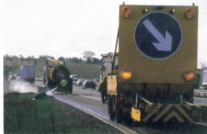
Reducing safety risks on highway works sites was discussed at a special seminar last month
